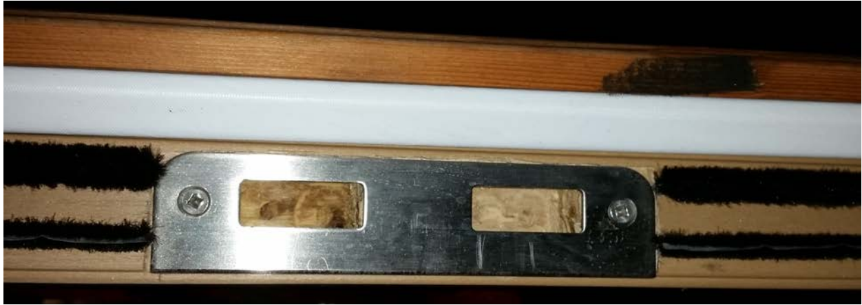
Lengths of weather-stripping on strike side of Panel 3
